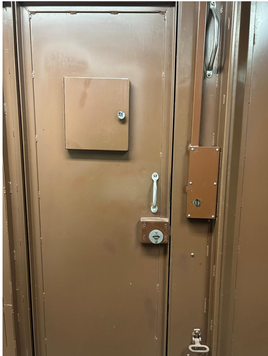
AGING DETENTION EQUIPMENT
