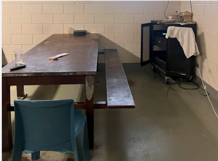
Poor Natural Light
