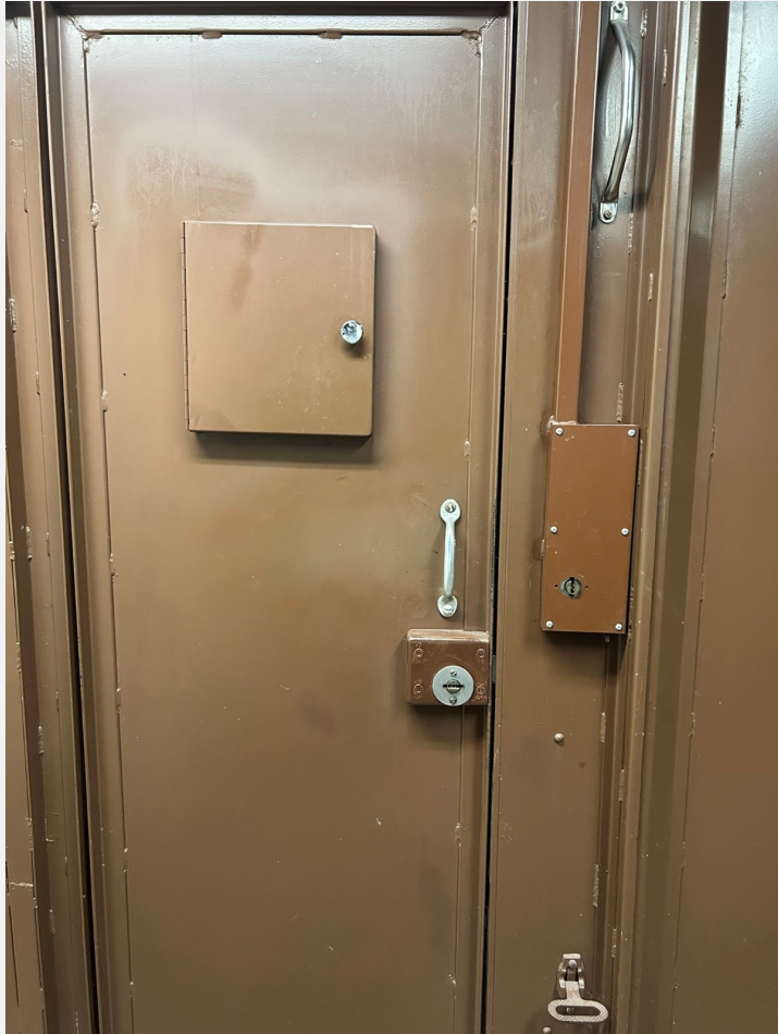
Aging Detention Equipment
